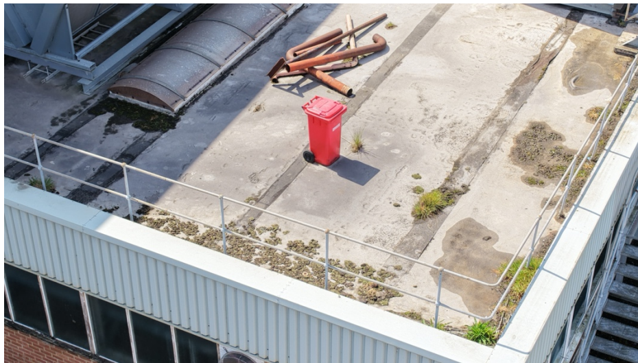
Figure 13. Biological Growth / Loose pipework
