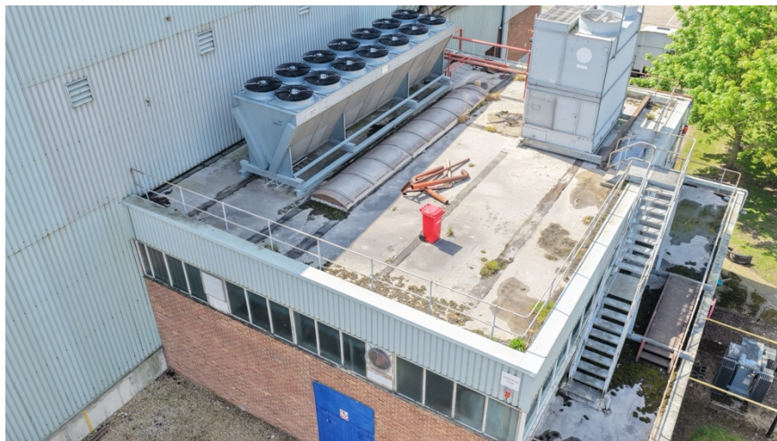
Figure 20. Vegetation and moss growth along plant deck edges and drainage areas.
