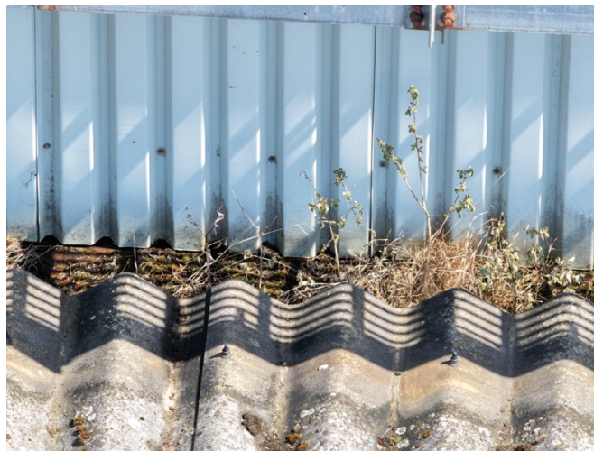
Figure 24. Dense vegetation around service penetrations indicating long-term moisture and sediment retention.
