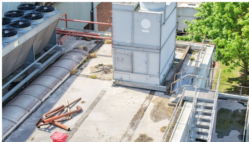
Figure 18 Loose redundant pipe sections and materials stored on the plant deck.
