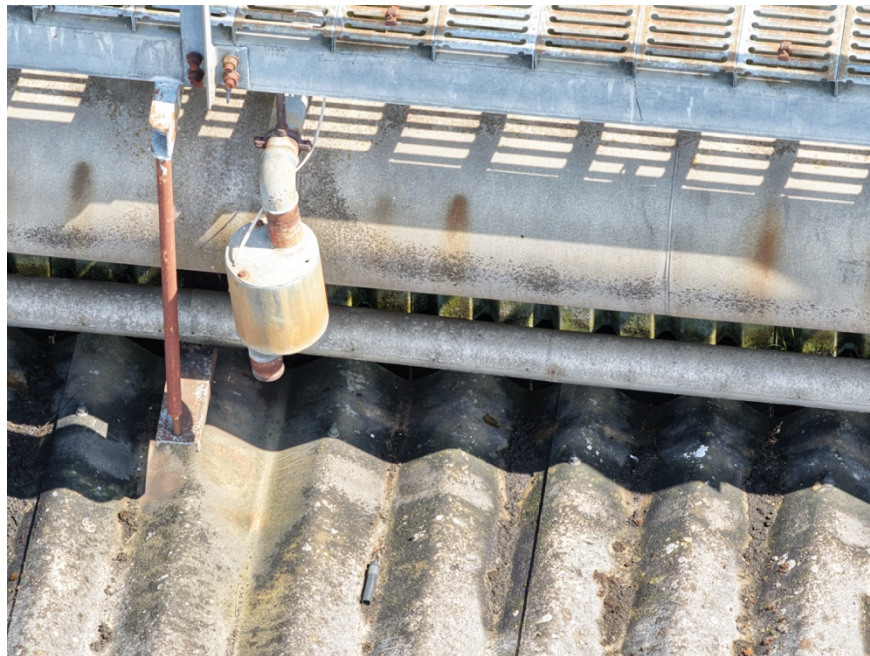
Figure 17. Corroded pipe support / service detail with deteriorated metal components.
