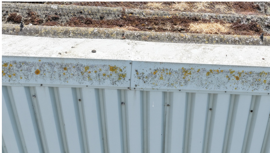
Figure 22. Biological growth, lichen and staining to perimeter capping.
