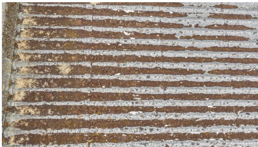
Figure 23. Localised roof sheet surface deterioration
