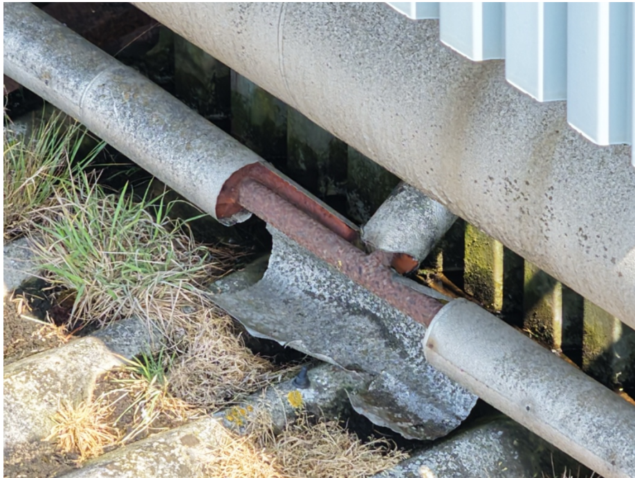
Figure 10. Corroded / Exposed pipework
