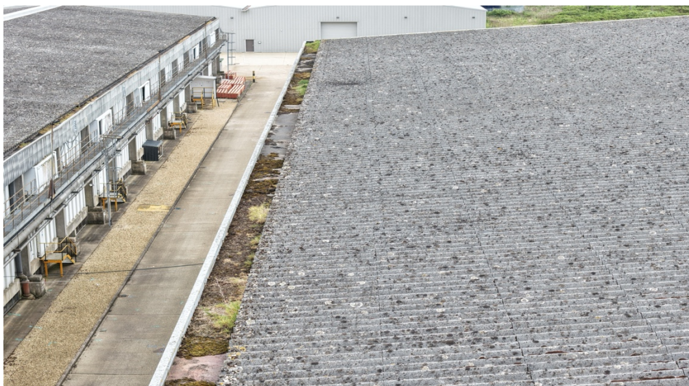
Figure 8. Corrugated roof sheet condition / Drainage issue
