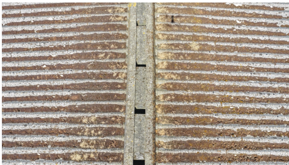
Figure 14. Widespread organic debris retained within corrugated roof sheet valleys.
