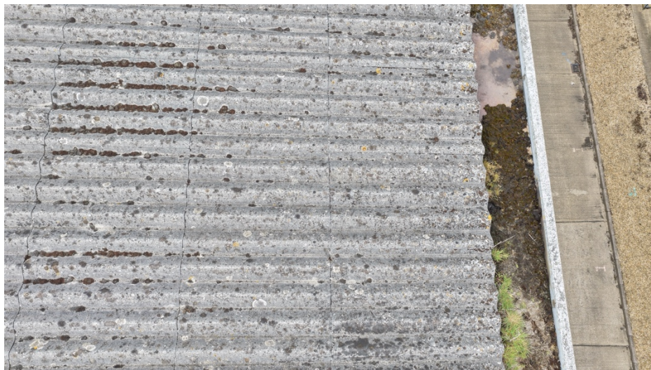
Figure 15. Restricted drainage channel with moss, sediment and vegetation at the roof-to-wall junction.
