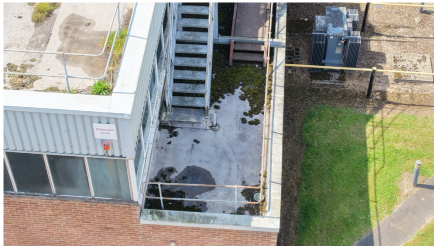
Figure 19. Standing water and moss accumulation around the access stair and lower plant deck area.
