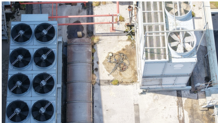
Figure 25. Loose cables, redundant materials and staining around plant equipment.
