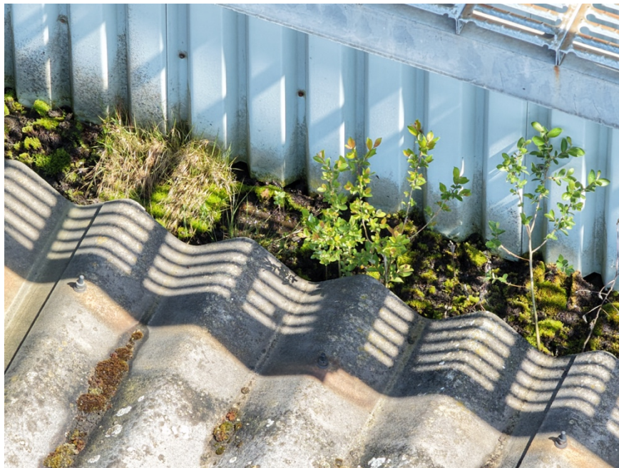
Figure 16. Established vegetation growth at the joint flashing and cladding base interface.
